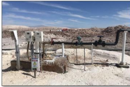
Figure 13-1. Field Pictures of a Typical Salar de Atacama Brine Production Well, Pipe, and Gathering Pond
